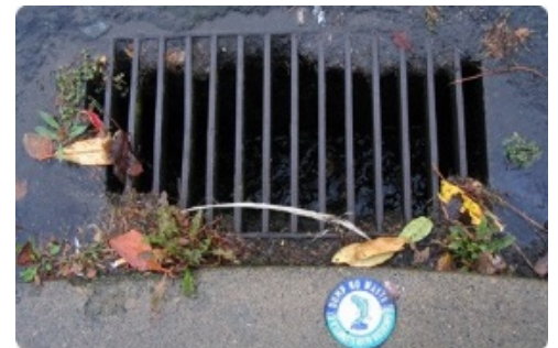
Catch basins drain stormwater directly into local waterways.
